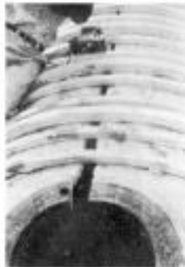
Burst pipe in power
